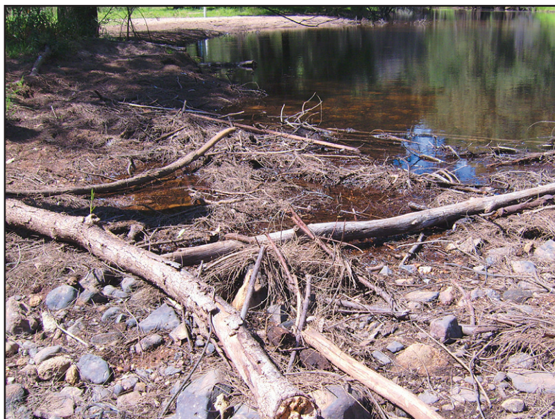
Example of a leaky weir.
